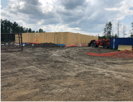
Work got underway quickly on the new Gordondale Hall once the ground was officially broken.
