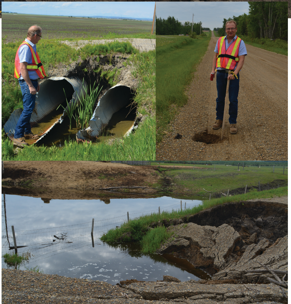
The County experienced extensive damage to its road infrastructure during the spring flood of 2018.
